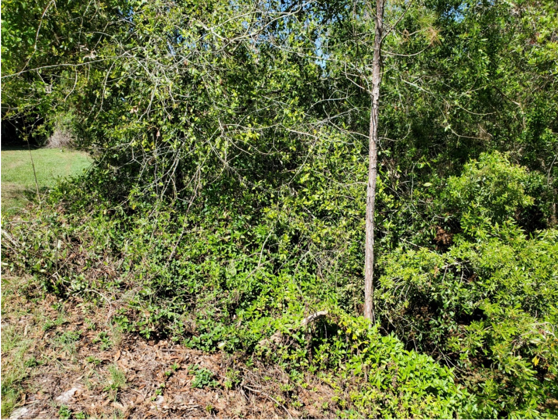
Complete vegetation overgrowth of the ditch area.
