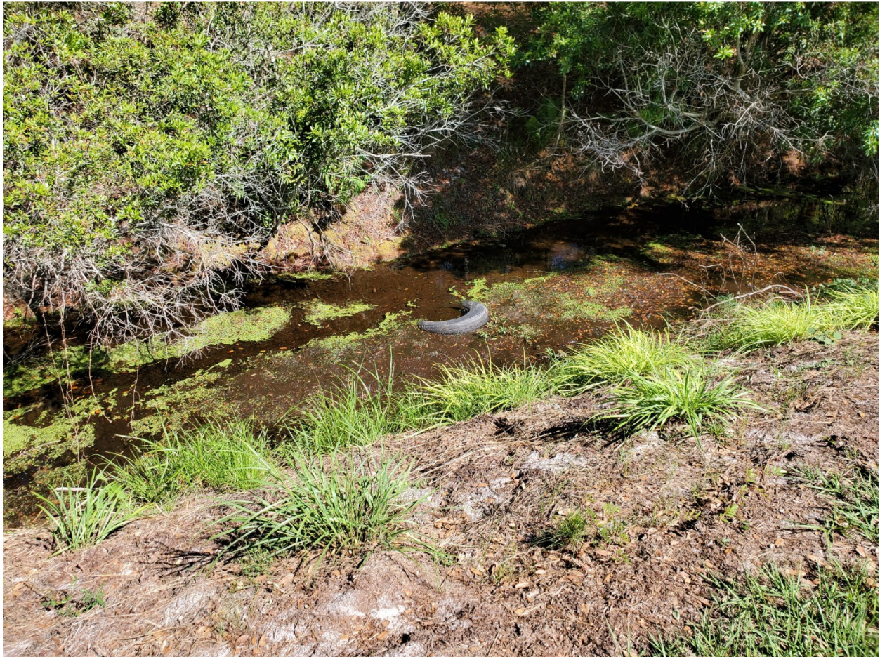
A tire is in the bottom of the ditch in the picture above. This was not the only instance a tire was seen in the ditch bottom.
