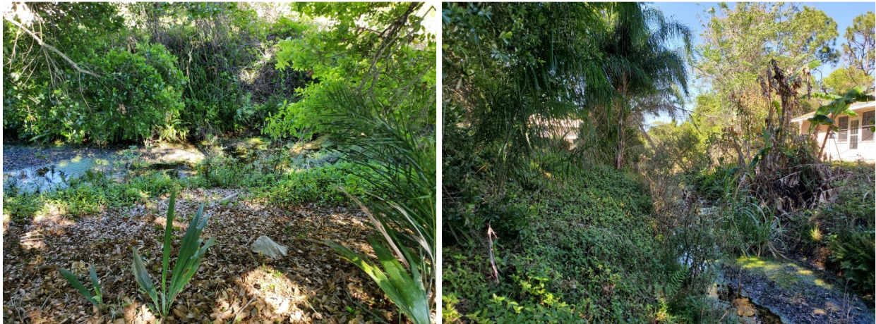
Moderate overgrowth of the ditch area as well as silting and build up in the ditch bottom.
