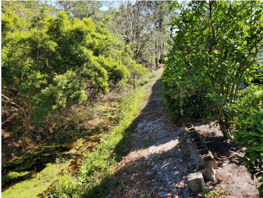
This picture depicts the area of the ditch near Fairway Road. Vegetation is more prevalent on the Sebring Hills side of the ditch than the Golf Hammock side. The bottom has signs of silting in.
